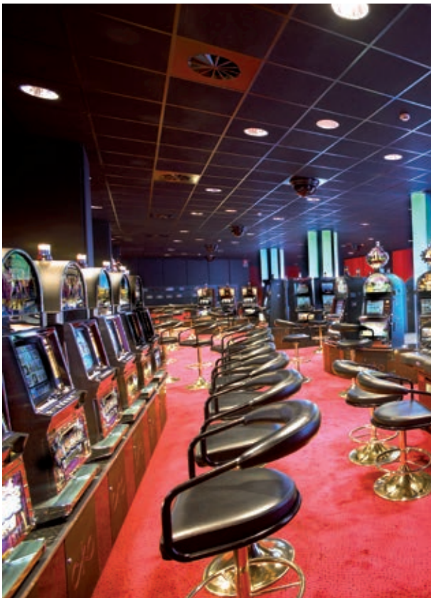
Radial outlet with square face in a casino
